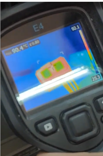
Back of Board observed through Thermal Camera
